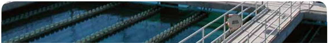
INDUSTRIAL WATER (FILTRATION) SYSTEMS
